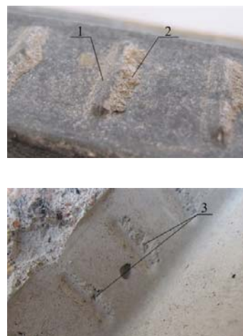
Fig 6. Nature of cutting of edge concrete keys: 1 – ribs of sheeting; 2 – edge of concrete keys; 3 – draw out edge of concrete keys
