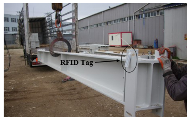
Fig. 4. Steel assembly with an RFID tag
